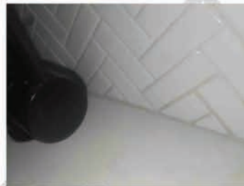
Cracked and deteriorated caulking observed around sink.
