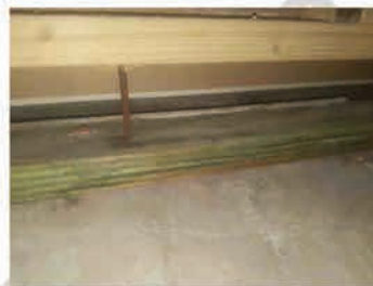
Water staining and damage observed on sill plate.
