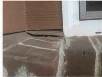
Openings and cracks observed.
