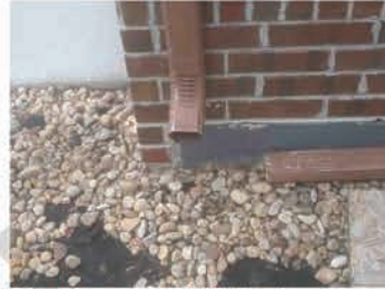
Downspout observed discharging at foundation.
