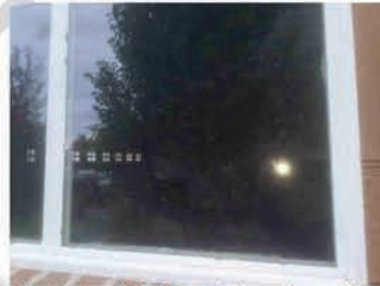
Cracked and broken window observed common Garage.
