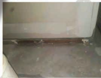
Water staining and damage observed on drywall and sill plate.
